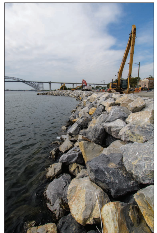
New sea wall being installed at Dennis Collins Park in Bayonne is a part of PPG's remediation activities.
